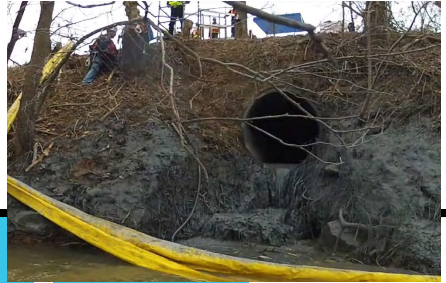
Failure in an abandoned pipe
